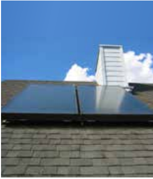
Vitosol 200-F flat plate solar collectors
