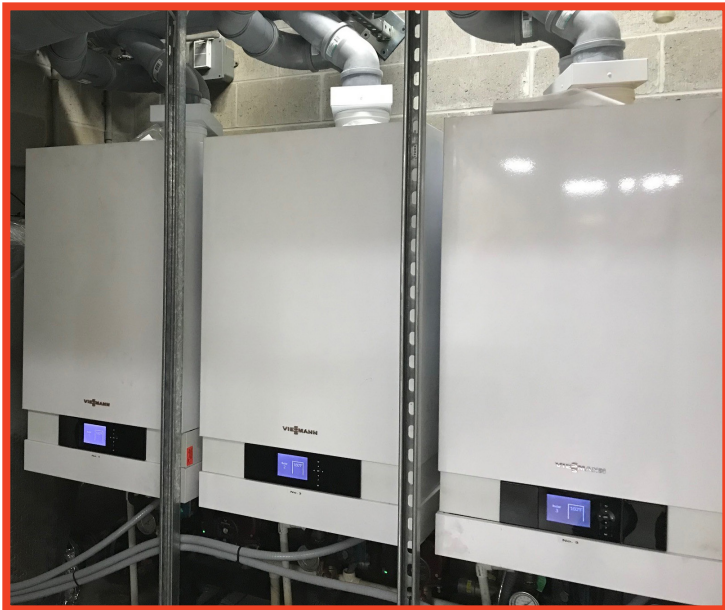
Vitodens 200 Cascade System provides heat for multiple pools at the Sturgeon Bay YMCA
