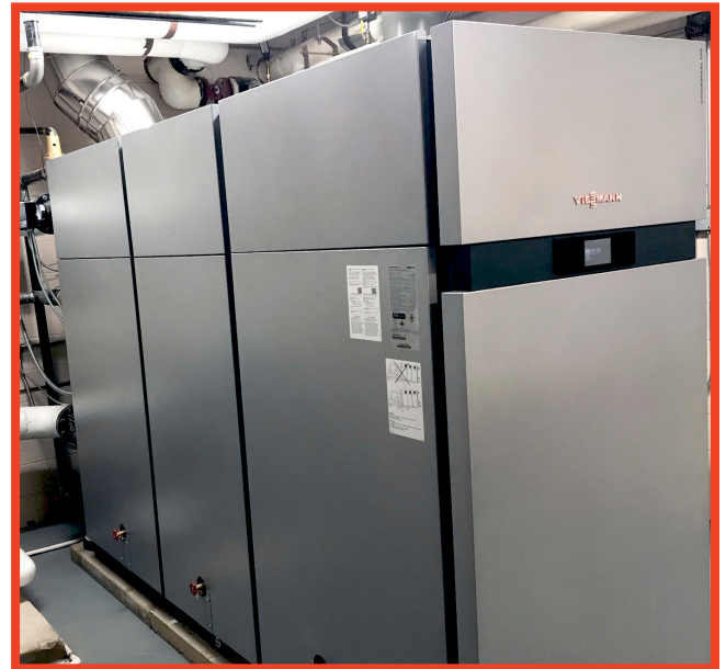
A single Vitocrossal 300 CA3B Provides complete space heating and DHW for the entire facility.
