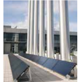
Large-scale horizontal Vitosol 200-F installation
