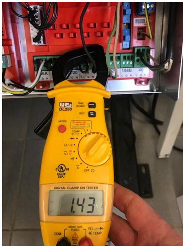
Measure Amperage to check Circulator Functionality
