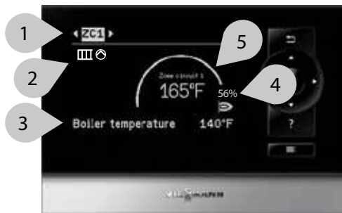
ZC Fixed Setpoint Configured
